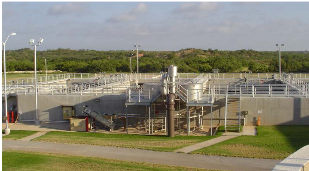
Waste Water Treatment Plant
