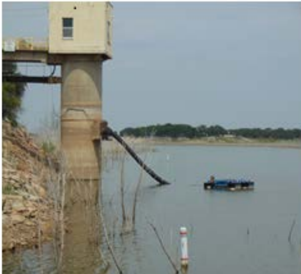
Oak Creek Lake – Surface Water Source
